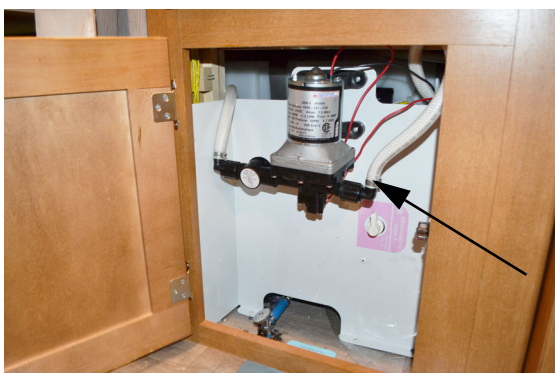
Water Pump (Located behind access door in bottom of pantry) *Models 22M -Typical View
