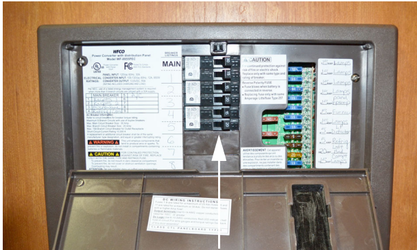
120-Volt Circuit Breakers -Typical View
